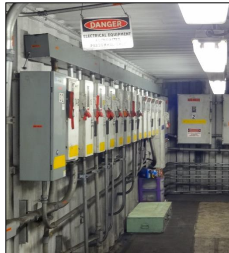
P8 Mine Electrical Panel Room
